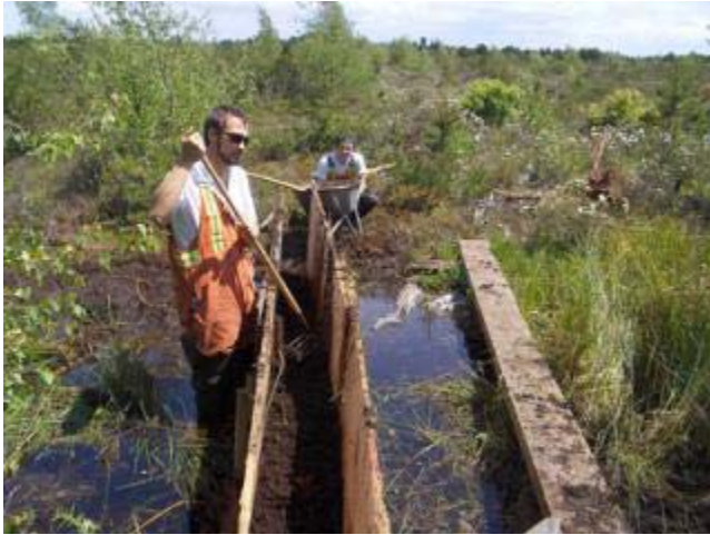
Restoration workers Mike Jeffery (left) and David Randt use soil and plywood to dam one of the drainage ditches in Burns Bog. (Courtesy Corporation of Delta)
